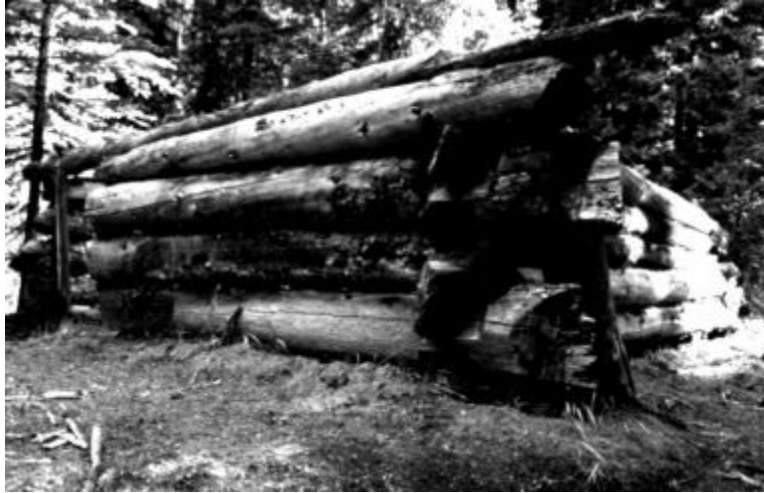
Figure 2. Picture of the front or west wall of the Tangle Creek Cabin.
