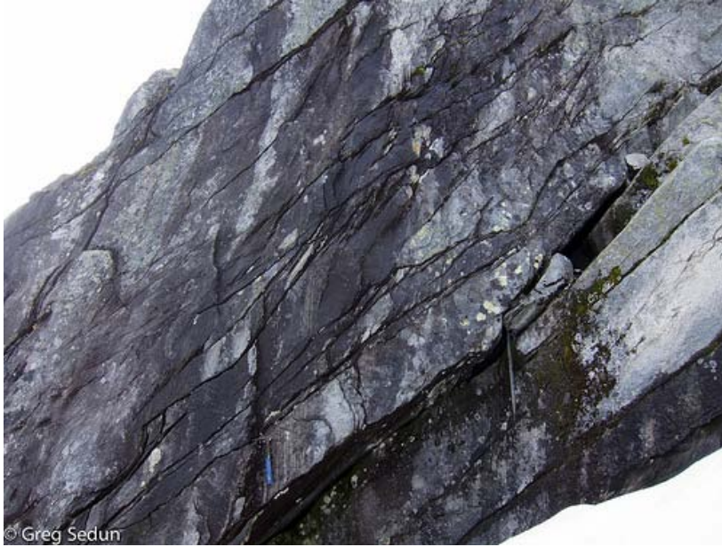
Figure 8. South wall of cirque illustrating the bottom and sidewall failure planes (blue handled rock hammer for scale) Source: Greg Sedun
